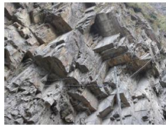
Figure 1. Lack of roughness and sufficient joint sets.
